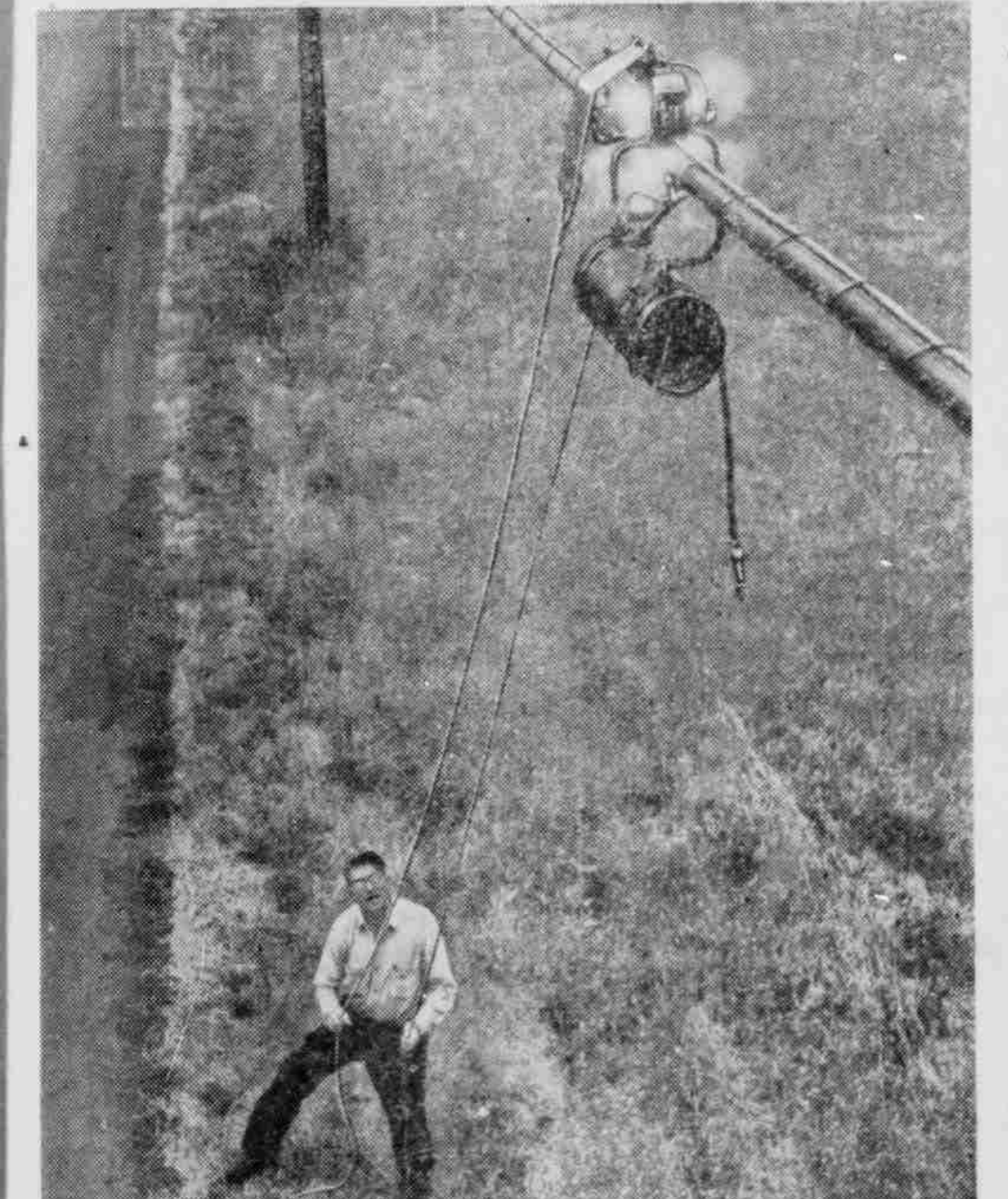
New sprayer fights cable-boring beetles. Astounding as it may seem, there's a kind of beetle that can eat right through the lead cover of a telephone cable. The beetle's so tiny it's hard to see. But the hole it leaves can let harmful moisture inside a cable. To prevent this, telephone people use a special repellent, which used to be brushed on cables entirely by hand. But the new sprayer—pulled by a man on the ground—puts the repellent on three times faster. By saving valuable time, this cuts the cost of guarding cables. So it's a big help in bringing you good telephone service that's high in value and low in price. Pacific Telephone works to make your telephone a bigger value every day.
