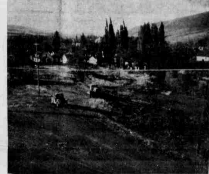
NEW SCHOOL SITE —The bulldozer had been working only a few minutes when this picture was taken Monday afternoon, but by Tuesday the area had an entirely different appearance as tons of dirt had been moved. The county is doing the excavation, and the building contract will be awarded separately. (GT Photos)
