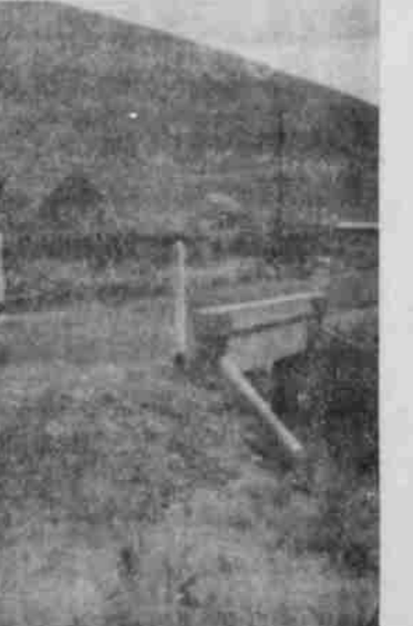
THE BRIDGE--this is the corner of the bridge into which most cars have crashed. It is of the same design and distance from the road as many others on the road. (GT Photos)
