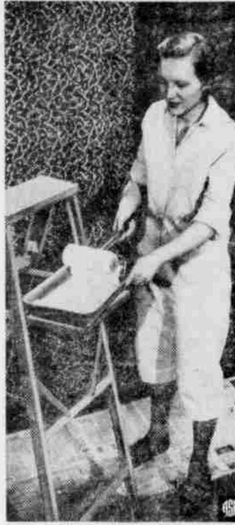
Applikay, picked up from the paint tray by the fabric roller, is transferred to the plastic design roller as the latter is rolled against the wall. Design shown is Silken Fleece.
