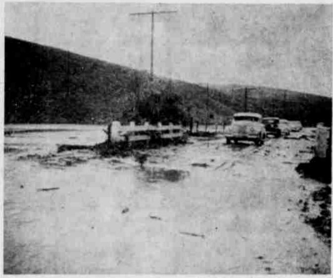
MUDCOVERED HIGHWAY at the mouth of Sourdough canyon between Lexington and Heppner is pictured here after the waters had receded during last Friday's waterspout. Just below this spot the waters washed a railroad bridge out of line necessitating repairs before trains could again cross it.
