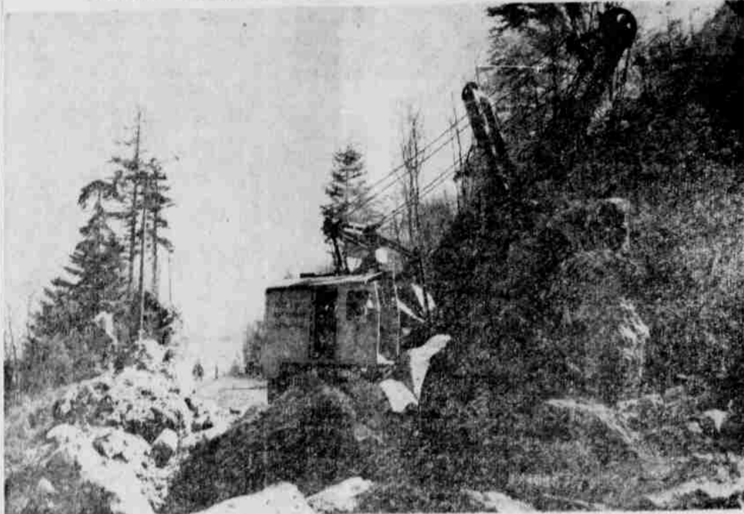
In the days of Samuel Lancaster and the other Highway Pioneers, the scenic loops and curves and grades of the Columbia Highway were built far above the river, with picks and shovels, freenas, mules and men; also black powder, star drills and a sledge. But, when the Moderns ironed out the curves, they did the grades down along the water-route and blasted their way through the foot of the bluffs, they did it with huge suction dredges, dynamite, bulldozers and dield oil. They made the barn-sized boulders into base material to fill the low spots until now you never feel a bump when you ride the road between Dodson and Bonneville where the boulders blocked the way when the above picture was taken. Construction like that costs approximately a third of a million dollars per mile.
