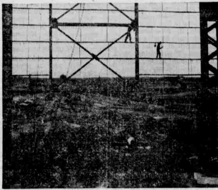
NEW STEEL FACILITIES TAKE SHAPE—Workman painting braces on the end of a new open hearth building. This new plant is part of the National Production Authority's program for the expansion of basic industry. It will play a major part in raising our steel capacity to 120 million ingot tons by the beginning of 1953.
