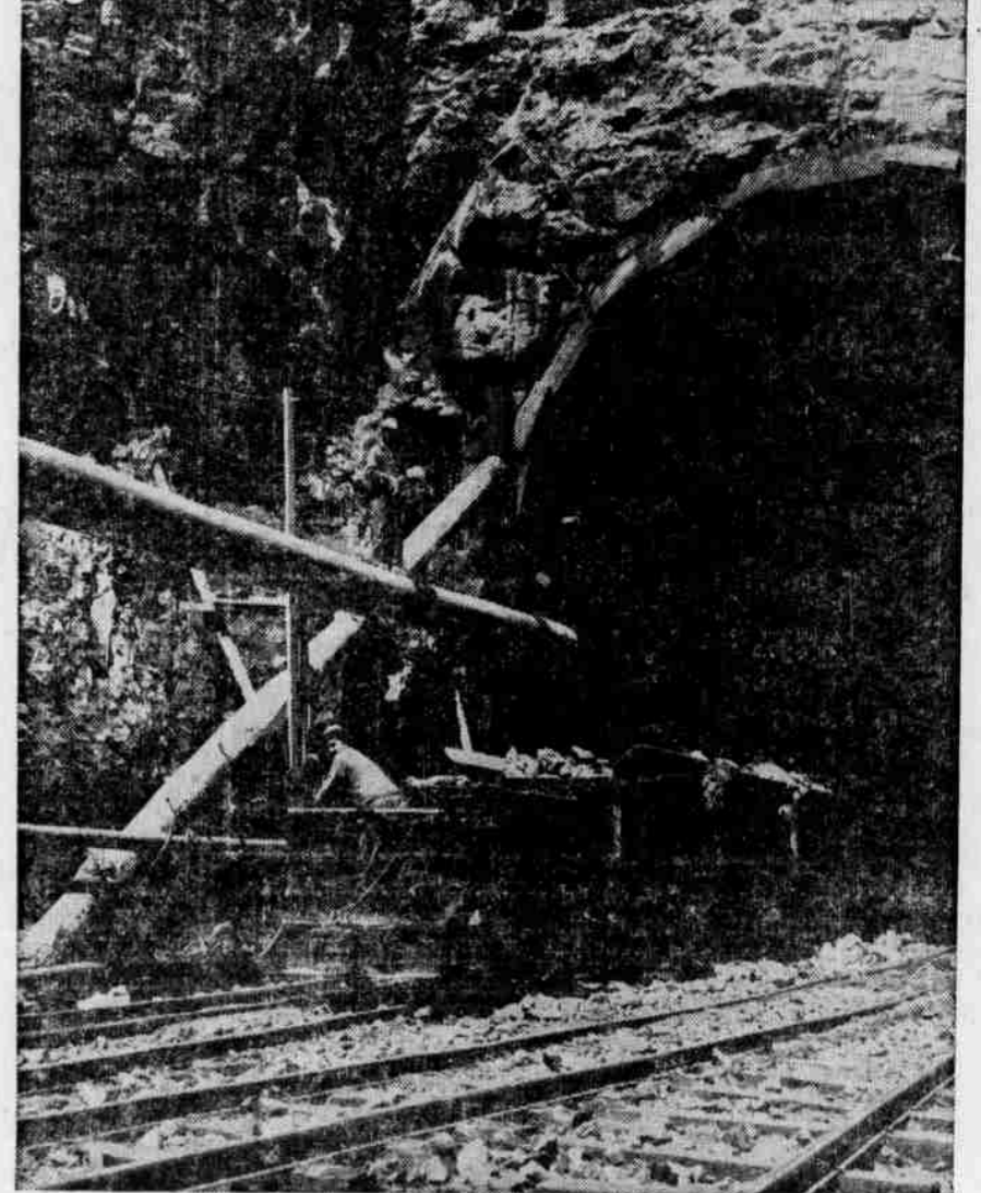
DIVERSION TUNNEL is being driven 1500 feet through solid rock. Lewis River will flow through this 30-foot-high tunnel while dam and powerhouse are being built.
