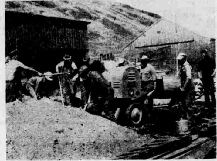
One of the Mixing Crews building. The work was streamlined so that no workman or busy it required two concrete group of workmen got in the way mixers, one on either side of the other groups.
