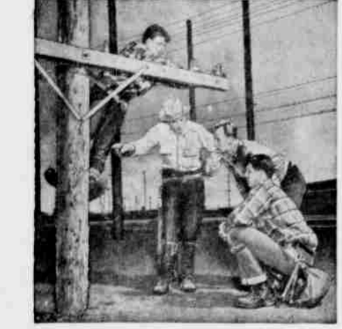
2. On stubby poles like these, linemen learn to use their new climbing equipment. This is just one of the more than one hundred courses that telephone people study in towns large and small—up and down the Coast. In 1948, thousands of employees received training. That means thousands of men and women better able to furnish good service to you.
