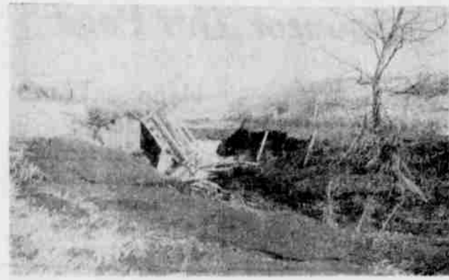
As evidence of what the run-off in February did to some of the roads, Judge J. G. Barratt snapped this view of the bridge above the John Graves ranch in Sand Hollow. Places where it has been convenient to replace the bridges the road crew has graded out new crossings.
