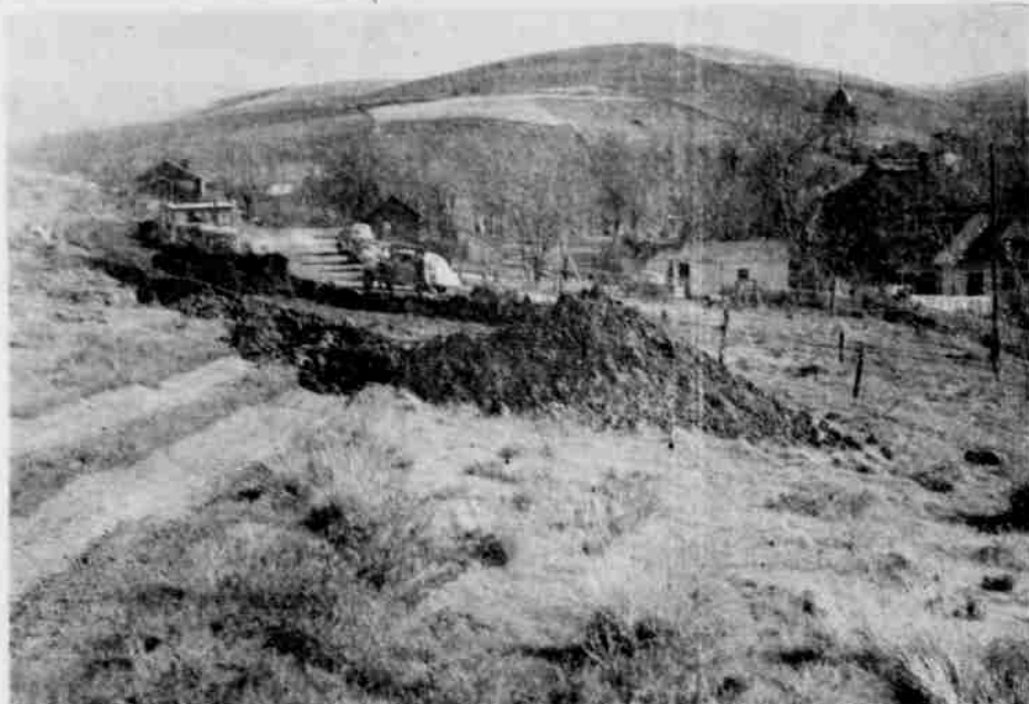
This is a view of the Barratt project work taken from the opposite end of the fill from the view on page 1. The work started the first day was carried out
