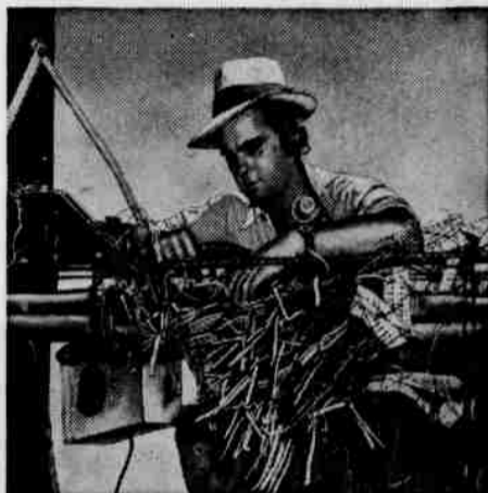
2. Complex splices like this—thousands of them—went into the two million miles of wire we've put in. And that's only part of the story—more than 200 new buildings or additions... complex new switching equipment in almost all our buildings... these and other facilities are being added in the face of sharply rising costs and tough supply problems.
