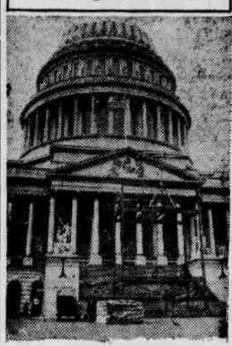
The partially completed inaugural stand in front of the Capitol where Herbert C. Hoover will take the oath of office as the thirty-first president of the United States.
