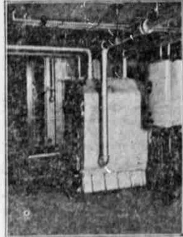
Burner Mechanism Almost Entirely Within Furnace.
