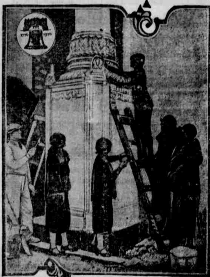
Young women artists turn from their jars of color and paint brushes to assist plasterers in setting ornaments in place atop huge pylons which adorn the main entrances to the Palace of Agriculture and Food Products, of the vast exhibition buildings which forms a part of the great Sesqui-Centennial International Exposition being staged in Philadelphia from June 1 to December 1 to celebrate the 150th anniversary of the signing of the Declaration of Independence. Climbing ladders and walking along rickety scaffolds is nothing new to these young ladies, but each time they do it they get a thrill.
