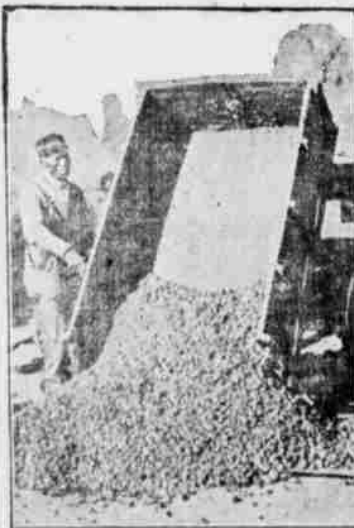
Truck Lead of Hot Bituminous Concrete Being Dumped Ready to Be Placed on Surface.
