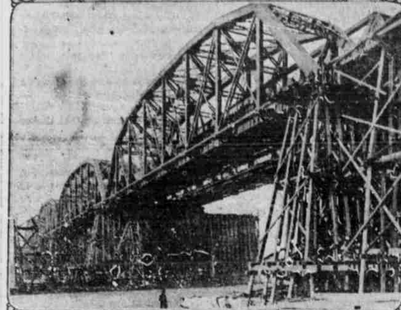
The old railroad bridge over the Missouri river at Omaha had to be changed for a new structure without holding up traffic too long. At the left (top picture) is the old structure, which was moved out of the way and the new one (at the right) put in its place in one hour. Lower picture, the two bridges.
