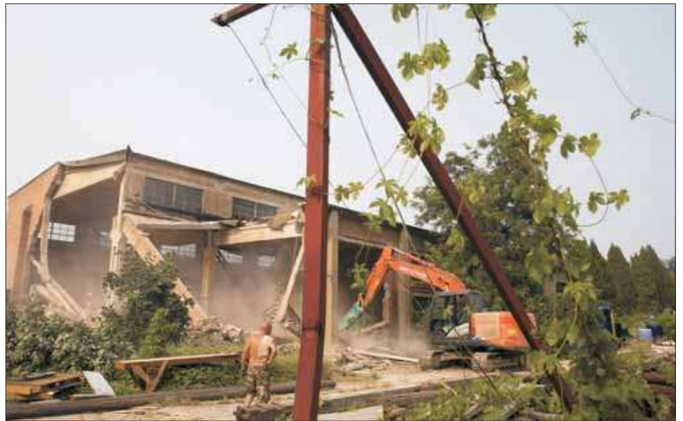
WORKSPACE WRECKED. Workers dismantle pipes (top photo) near artworks in Chinese artist Ai Weiwei's studio, which was demolished (bottom photo) in Beijing in early August. The frequent government critic said on his Instagram account that the demolition began without prior notice and posted videos of an excavator smashing the windows of his "Zuoyou" studio. (AP Photo/Ng Han Guan)
