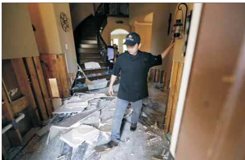
DISPLACED AGAIN. Viet Dao walks through debris in the foyer of his home in Spring, Texas. As Hurricane Harvey's flood water rose quickly above cabinets, counters, and toward the ceiling, he scrambled to figure out how he would save his young children, wife, and in-laws if the water would not stop. (AP Photo/David J. Phillip)
