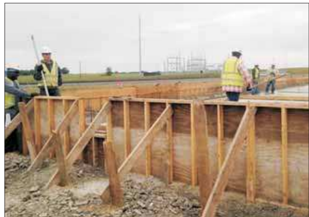
FROM PASTURE TO TIRE PLANT. Workers help construct a terminal to unload oil from rail cars at the $300 million Yokohama tire plant in West Point, Mississippi. The state of Mississippi borrowed $70 million to help finance improvements, including a rail spur used to deliver raw materials to the unit of Japanese tire maker Yokohama Rubber Co. (AP Photo/Jeff Amy)
