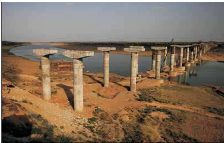
SURVIVAL OVER CONSERVATION? A bridge is seen under construction on the Chambal River near Sagarpada in the western Indian state of Rajasthan in this April 30, 2014 file photo. A narrow 250-mile stretch of the Chambal was declared an official sanctuary in the late 1970s, closing it to everyone except longtime villagers, approved scientists, and the handful of tourists who made it here. But with India's economic growth came troubles that threaten the Chambal and its wildlife: polluting factories, illegal sand mining, and fish poachers who hack at gharials with axes when the animals get tangled in their nets. (AP Photo/Altaf Qadri, File)
