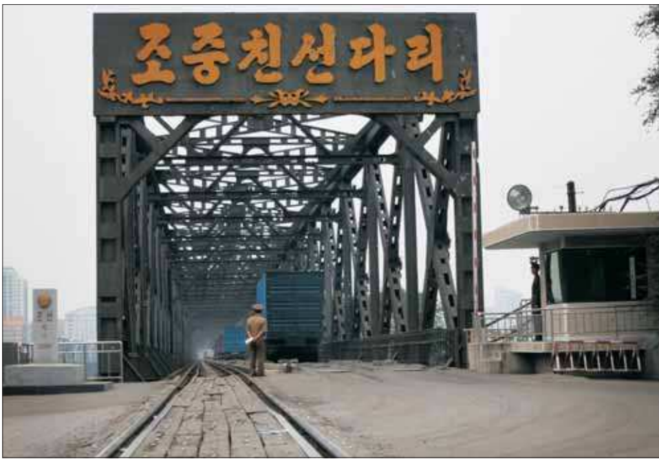
ONE-WAY INTEREST. This September 2, 2014 photo shows an entrance in Sinuiju, from North Korea to China using the "Korea China Friendship Bridge" — the old bridge connecting the two socialist states over the Yalu river. A new bridge that was built was supposed to be a key link for trade and travel between China's underdeveloped northeast provinces and a much-touted special economic zone in North Korea — so key that Beijing sank more than $350 million into the mammoth, three-kilometer-long structure that was slated to open this past fall. Now, it is beginning to look like Beijing has built a bridge to nowhere. The letters read: "Korea China Friendship Bridge." (AP Photo)
