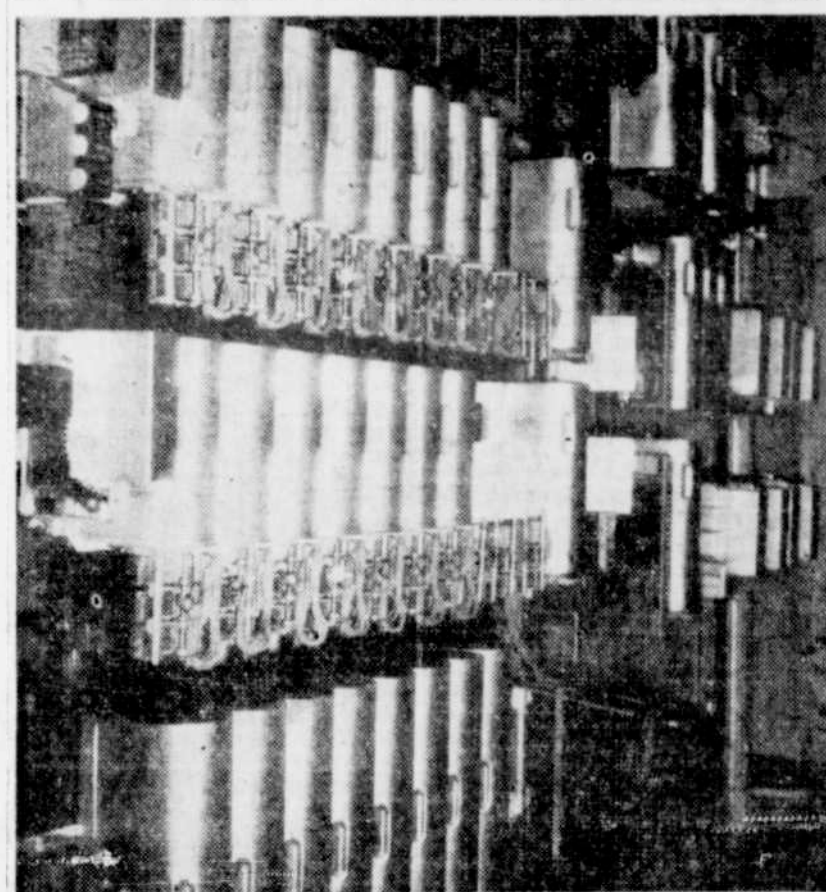
BEAVERTON. (Special)—This modern brick building in downtown Beaverton is the headquarters for the West Coast Telephone company's new dial system in this locality. Bottom view shows a portion of the mass of equipment which handles calls automatically.
