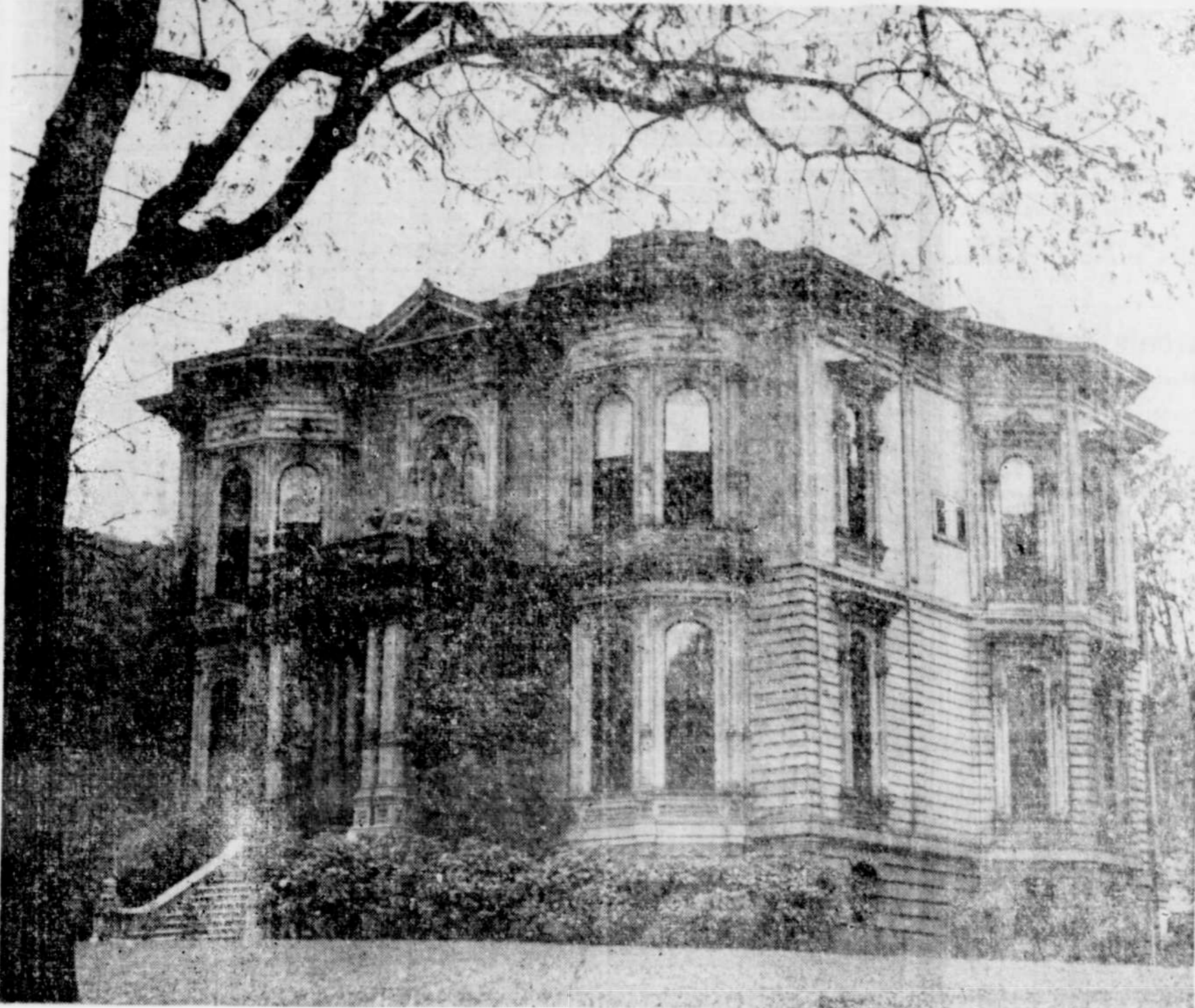
The Famous Jacobs residence S. W. Park and Montgomery st., now being wrecked by the Sunset Wrecking Co. Photo Courtesy Oregonian
