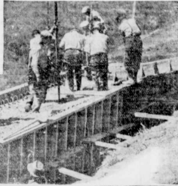
ABOVE—Southern California tunnel on Sepulveda boulevard. It gives access to the valley highway, No. 99, from south and west coast cities and resorts.
