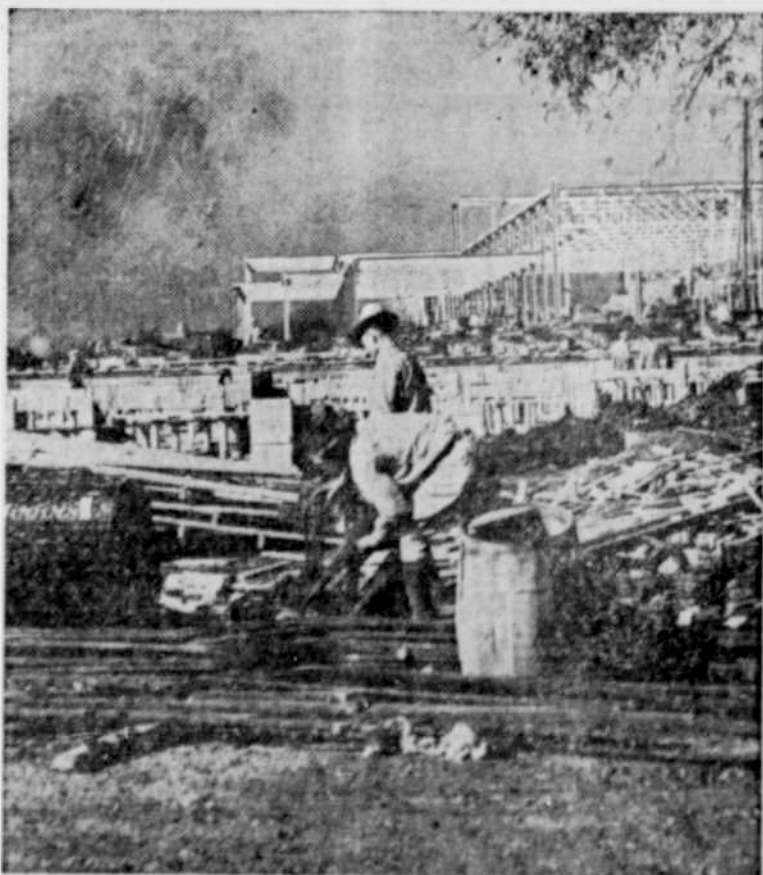
The steel frame of the $140,000 Livestock Building No. 2 for the Texas Centennial Exposition at Dallas can be seen above as it rapidly takes form. With the $260,000 Livestock Building No. 2, soon to be started, it will show the greatest exhibit of livestock in the nation's history when the Exposition opens June 6.
