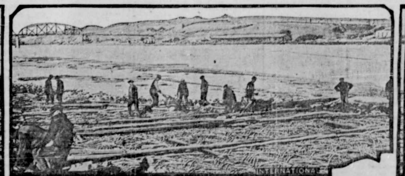
Workmen near Mandan, N. D., rip-rapping the banks of the Missouri river as protection against the expected spring freshets. The work consists of laying rock on willow mat and sinking it in the river. Liberty Memorial bridge is shown in the background.
