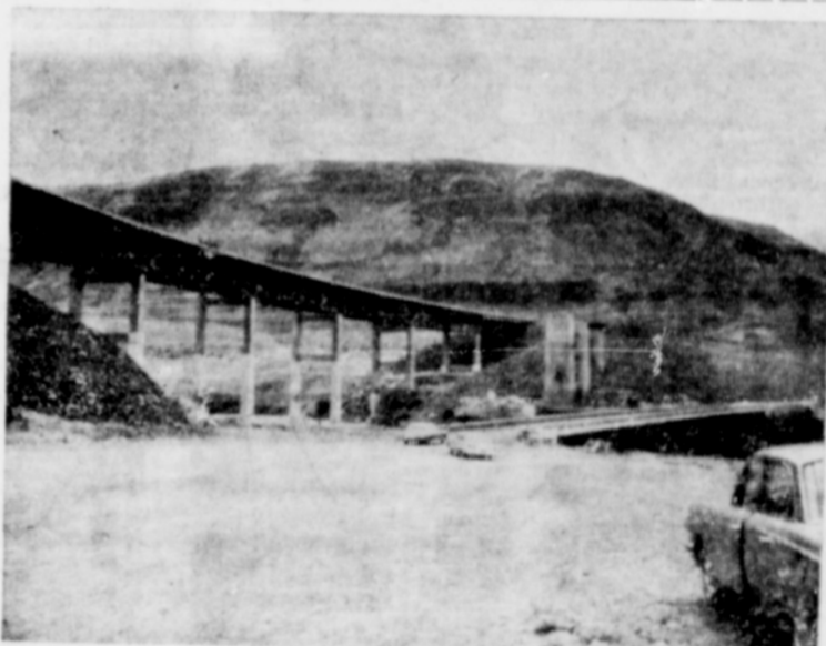
HIGHWAY 30 traffic will be directed soon across the new John Day River bridge pictured above. The bridge is part of the huge highway and Union Pacific Railroad relocation projects as a result of the construction of John Day Dam about two miles west of the mouth of the John Day River. The new highway bridge is approximately 150 feet higher than the Hwy 30 bridge which has been in use for many years.
