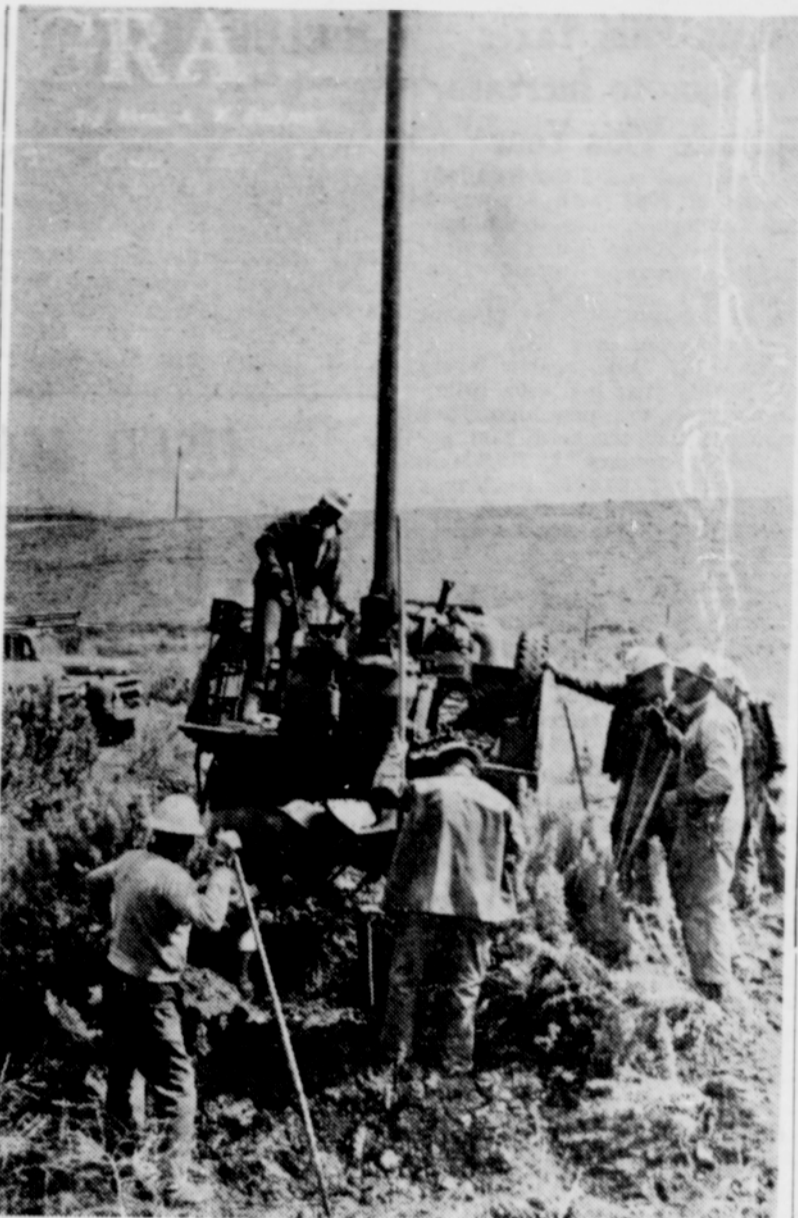
A TRUCK MOUNTED pole hole digger eliminates most of the pick and shovel work for P&L construction crews currently working on relocating the company's Moro-Wasco transmission line. Total cost of the project is an estimated $66,000
