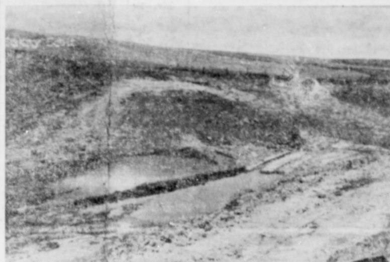
The beginning of a dam as a part of the soil conservation practices that won for Bill Todd the title of Soil Conservation Man of the Year for Sherman county. The dam is on an arm of Ferry canyon below the Todd buildings. Work had to be stopped due to wet weather but it will rise to about 20 feet within a month or two.
