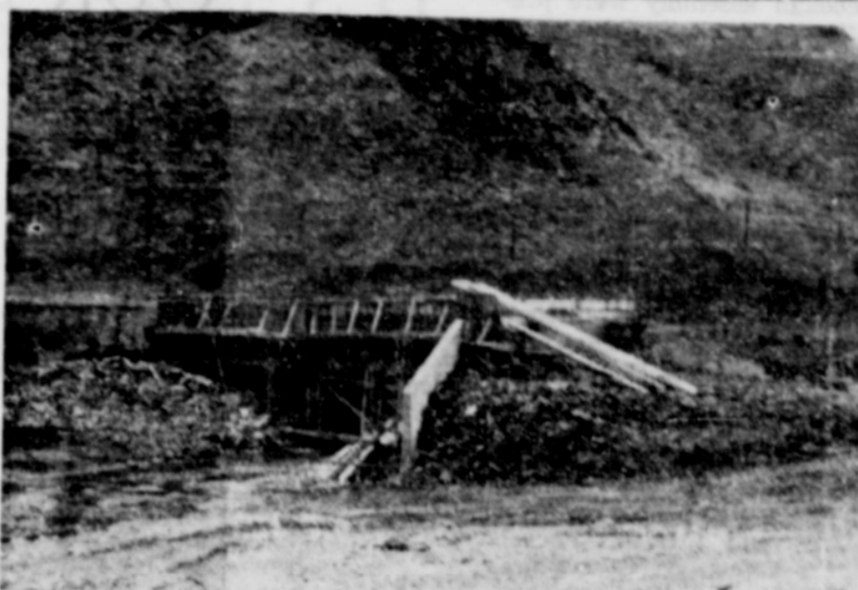
The road up Spanish Hollow is being rebuilt and it looks as if it will be much improved as to alignment. The road will be higher than before. Here is the new bridge across the creek to the Mud Hollow road.
