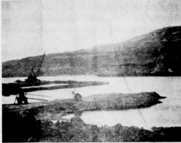
Right here will be the end of the John Day dam on the Oregon side. Crews are pushing gravel into the river to raise a base for the coffer dam that will be built later this year. And off to the left there will be a row of power houses and the water will rise over their spot higher than any building in the county.
