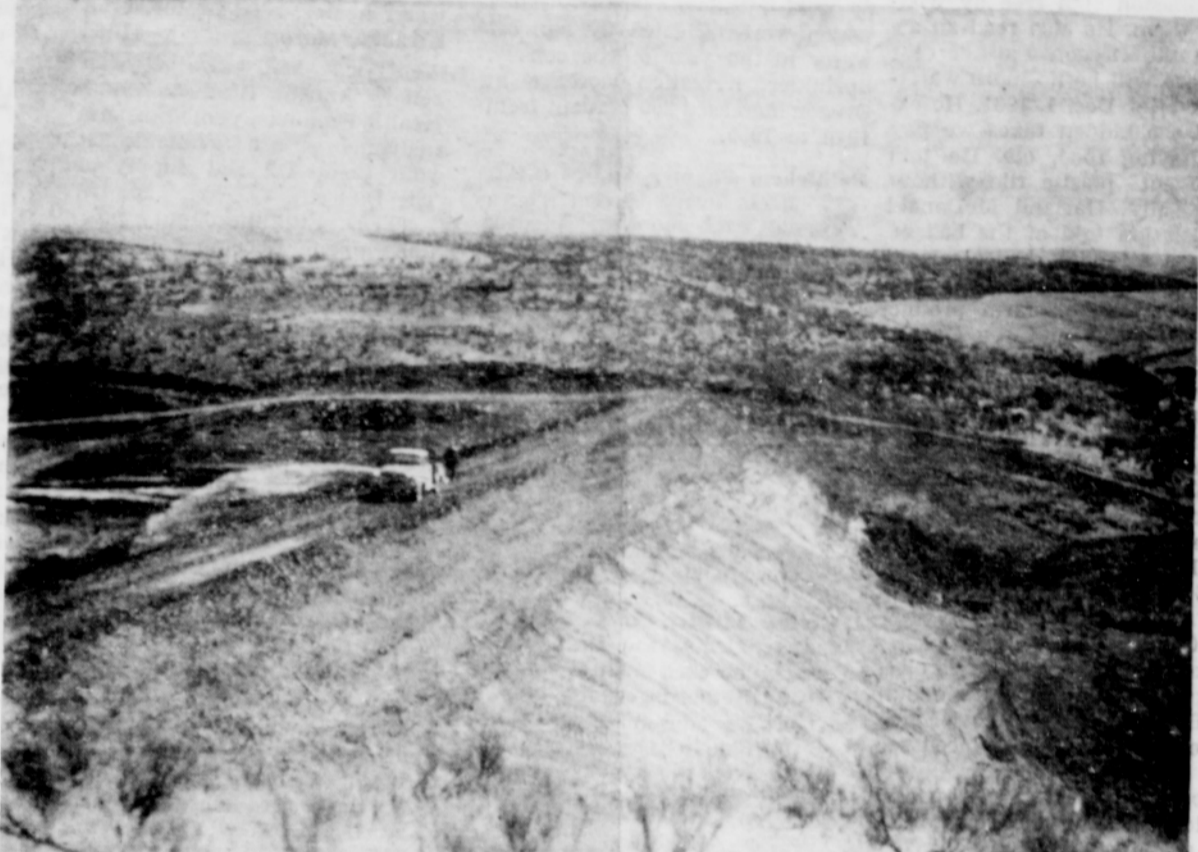
Joe Bibby's dam is nearly done after a summer of digging and bulldozing dirt and rocks around the Box canyon a half mile east of the Bibby home place.
