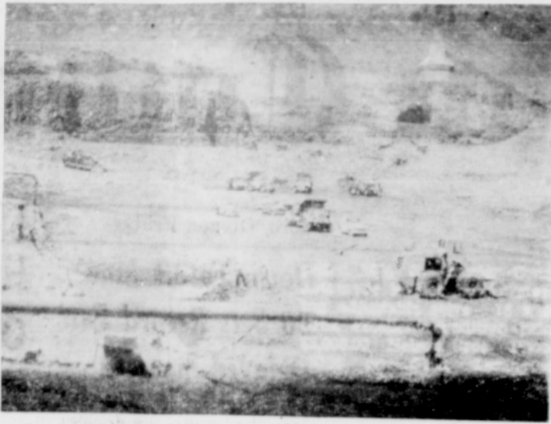
The picture isn't good but if you look sharp you may see the activity that went on at John Day dam a few minutes prior to the first concrete pouring. Men were washing all dirt off the base rocks with power hose, men were load- ing 34 yard dump trucks with lift vehicles, men were cleaning rock and sand from pockets. The big- gest machinery of its kind is at work there.
