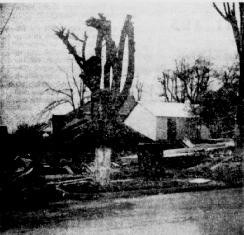
Before and after pictures showing the demolition of the two old buildings on the site of the new postoffice building. The McVicker Construction company did the wrecking and has the contract for the new building.
