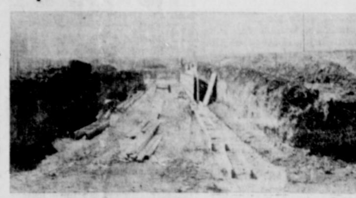
Above is the heat and utility tunnel which will run lengthwise of the new school building, from the heating plant under the gym at the south end to the music room under the stage at the north end. Camera was pointed south.
