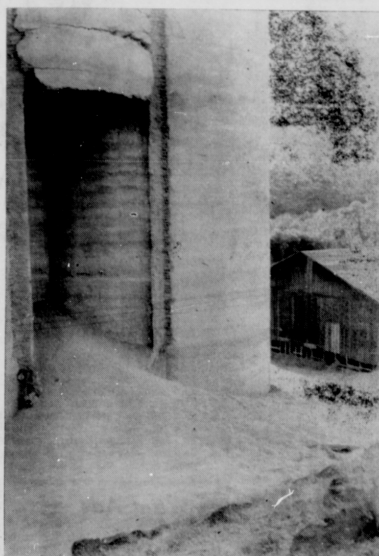
This picture of the broken convex, one side concave and one side straight. The upper elevator shows how the wheat part of the concrete work did spill out from pressure of its weight. Approximately 30,000 bushels were in the four sided removed bin, two sides of which were
