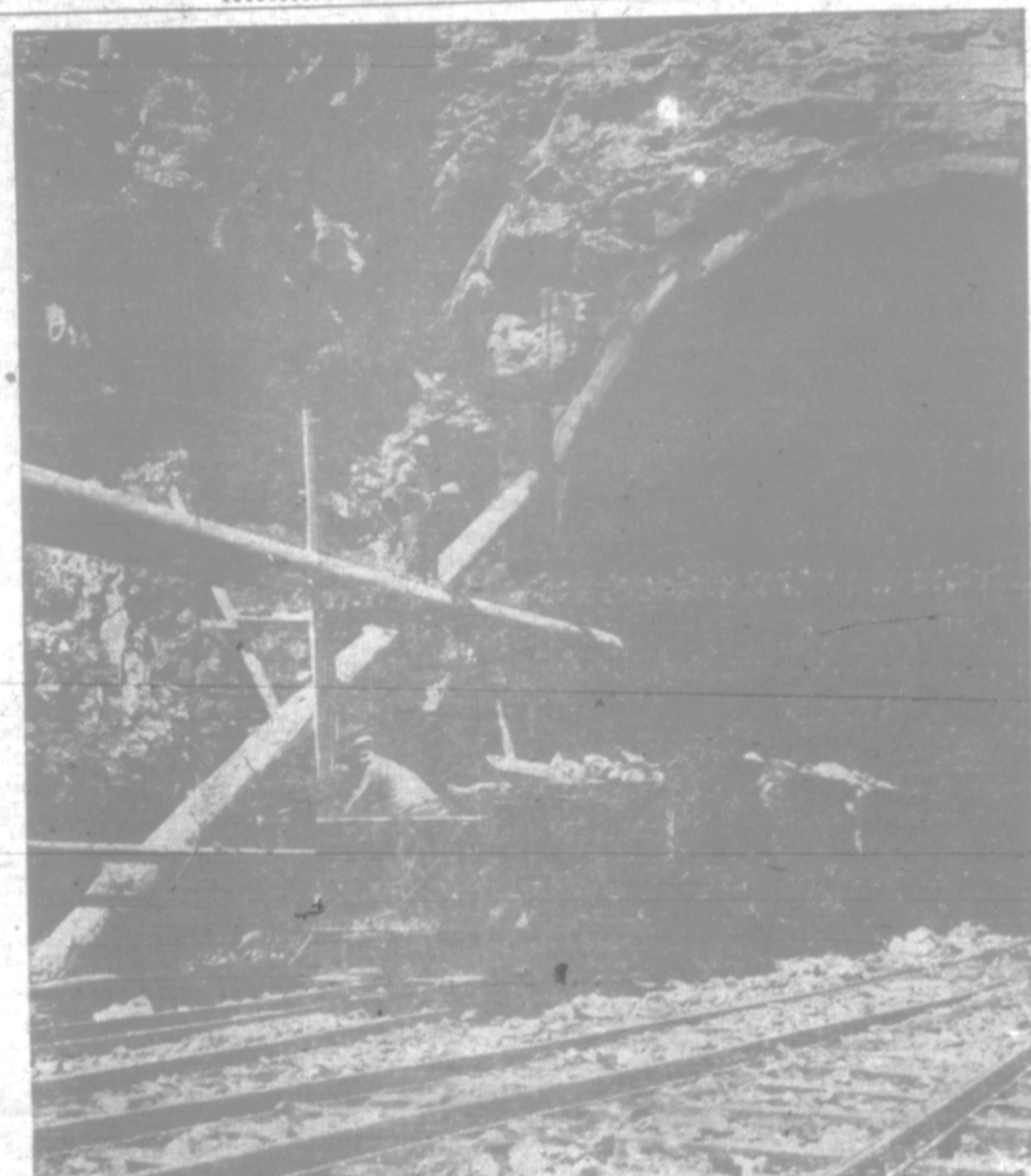
DIVERSION TUNNEL is being driven 1500 feet through solid rock. Lewis River will flow through this 30-foot-high tunnel while dam and powerhouse are being built.
