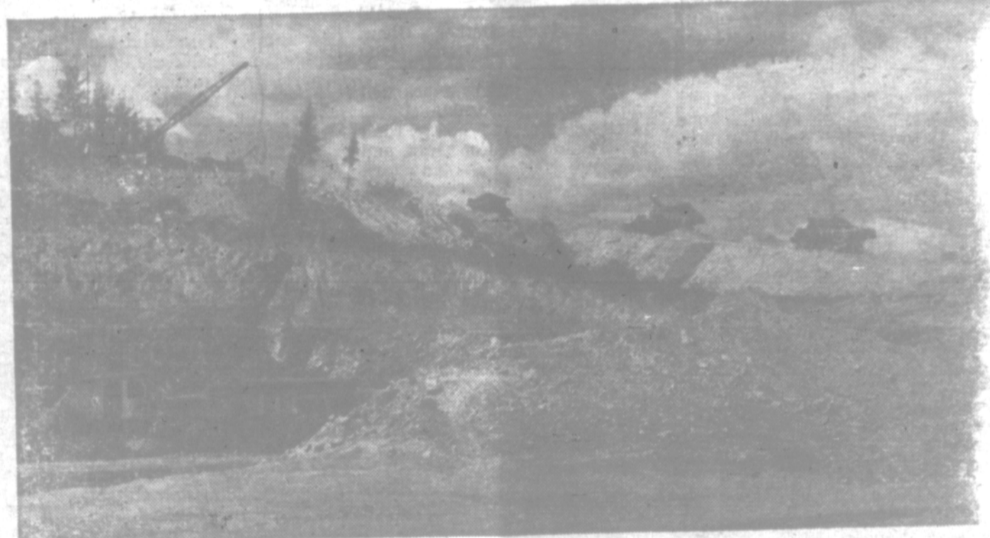
WORK AT MANY LEVELS prepares site for dam construction. Batteries of floodlights are used to illuminate the scene for night work. More than 3,000,000 cubic yards of rock and clay will go into the main portion of the dam. On completion, the main Yale dam section will be 300 feet high, 1500 feet long at the crest.
