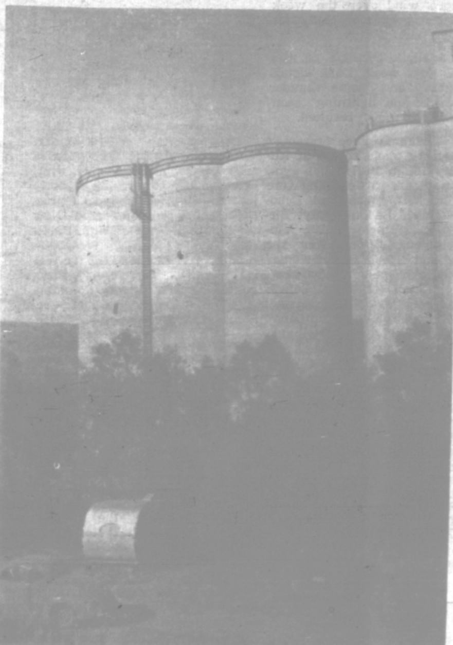
The new 400,000 annex to the Hay Canyon elevator is being finished in time to be filled by the new crop. Built by the Central Construction company crew it has two 47 foot bins, and a central series of bins.
