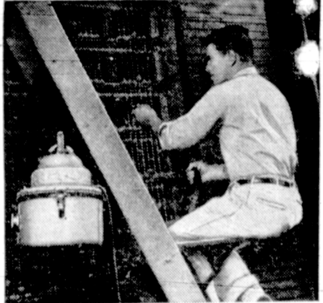
1. Imagine a vacuum cleaner in a central office... actually it's one of our important tools. For keeping equipment working perfectly means keeping equipment perfectly clean. The vacuum sucks up the specks of dust that might make a tiny electrical contact fail... just when you need it. And we stop trouble other ways, too.
