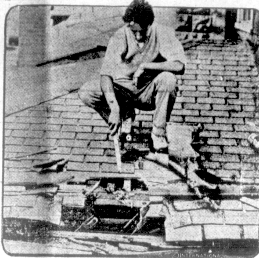
This man is pointing to the 14-inch hole that was torn in the roof of the home of Philip Schwab in Canasie, N. Y., when a bomb dropped by naval reserve aviators during practice over Canasie bay went wide of the target. Mr. and Mrs. Schwab and their two children were in the house when the bomb fell, but none was injured.
