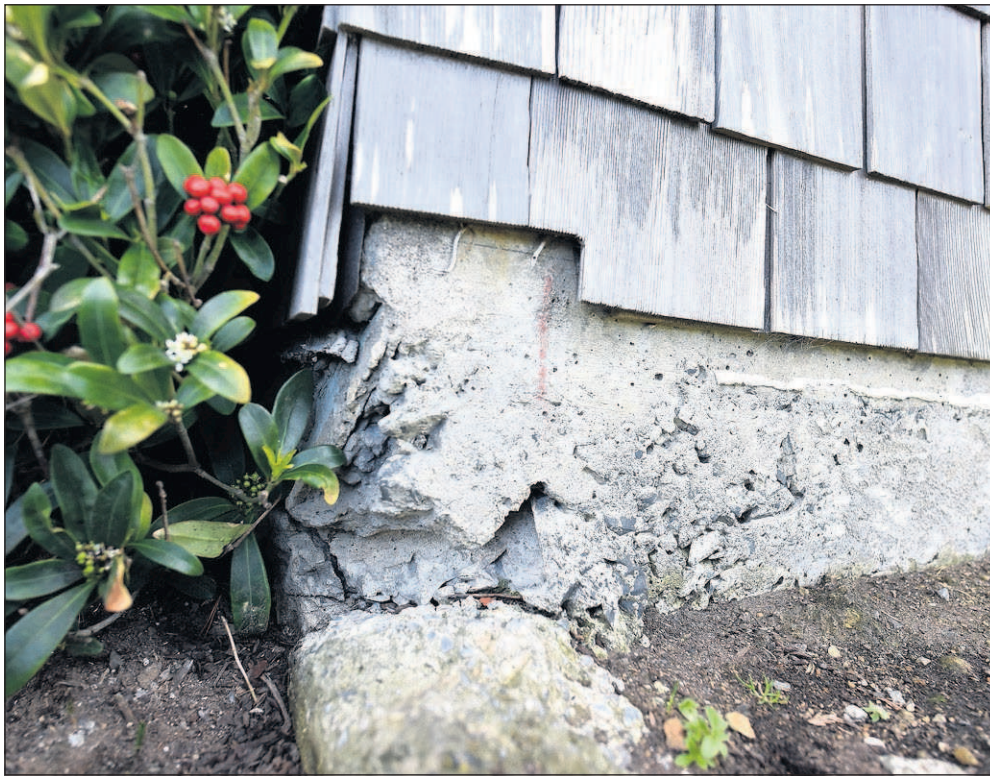
Damage can be seen to the foundation of the City Hall building in Cannon Beach.
