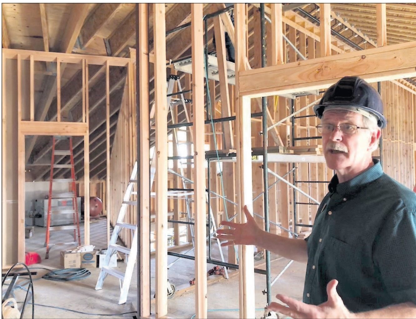
Jeff Carlsen gives a tour of the new construction at the center.
