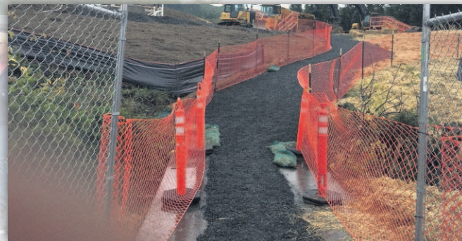
Access to the construction site for visitors at the school district's public groundbreaking.
