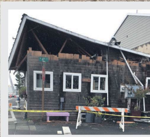
Damage along Laneda Avenue.
