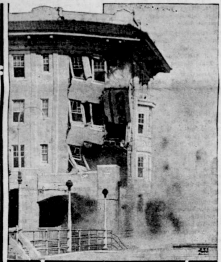
When the Hotel Brighton at Long Beach, N. Y., collapsed, a photographer was almost directly beneath it and, unmindful of the danger, he secured this masterpiece of news photography. Approximately $100,000 damage was done to the $1,000,000 structure, whose foundations were weakened by high seas.
