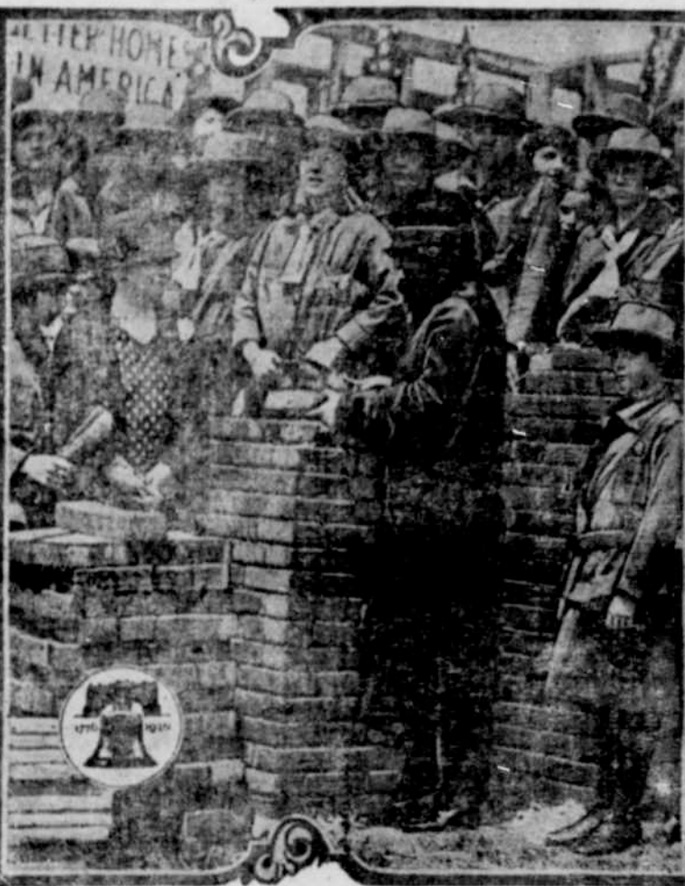
Mrs. Herbert Hoover, wife of the Secretary of Commerce in President Coolidge's cabinet, is shown laying the cornerstone for the model home being erected by Better Homes in America organization at the Sesqui-Centennial International Exposition, in Philadelphia, June 1 to December 1 to celebrate 150 years of American Independence. Opposite Mrs. Hoover stands Mrs. Vance McCormick of Harrisburg. The Girl Scouts grouped around the women will operate the house.
