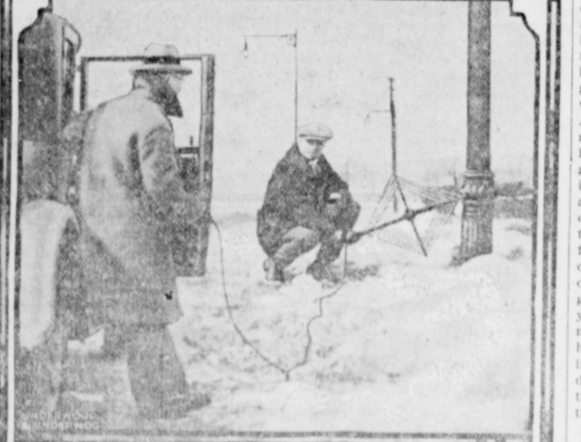
A crew of electrical experts in Revere, Mass., have devised a scheme whereby underground cable trouble can be located with the use of a radio outfit. Men are shown here attempting to find a severed cable that feeds lights on the Revere Beach boulevard. By carrying a loop antenna arrangement over the ground the trouble is found through a set built in the coupe.
