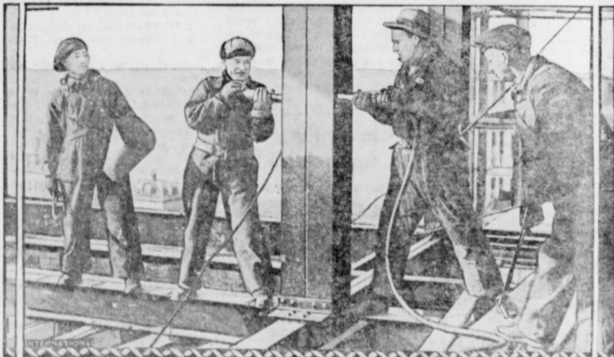
John Tarbell, Joe La Olaire, Jack Hill and Peter Horn, Iroquois Indians, formerly of the Kanawake reservation in Canada, who, having tired of the life on their reservation, have left it and are enjoying life by riveting on steel structures. They are at present working on the Columbia Presbyterian Medical Center in New York.
